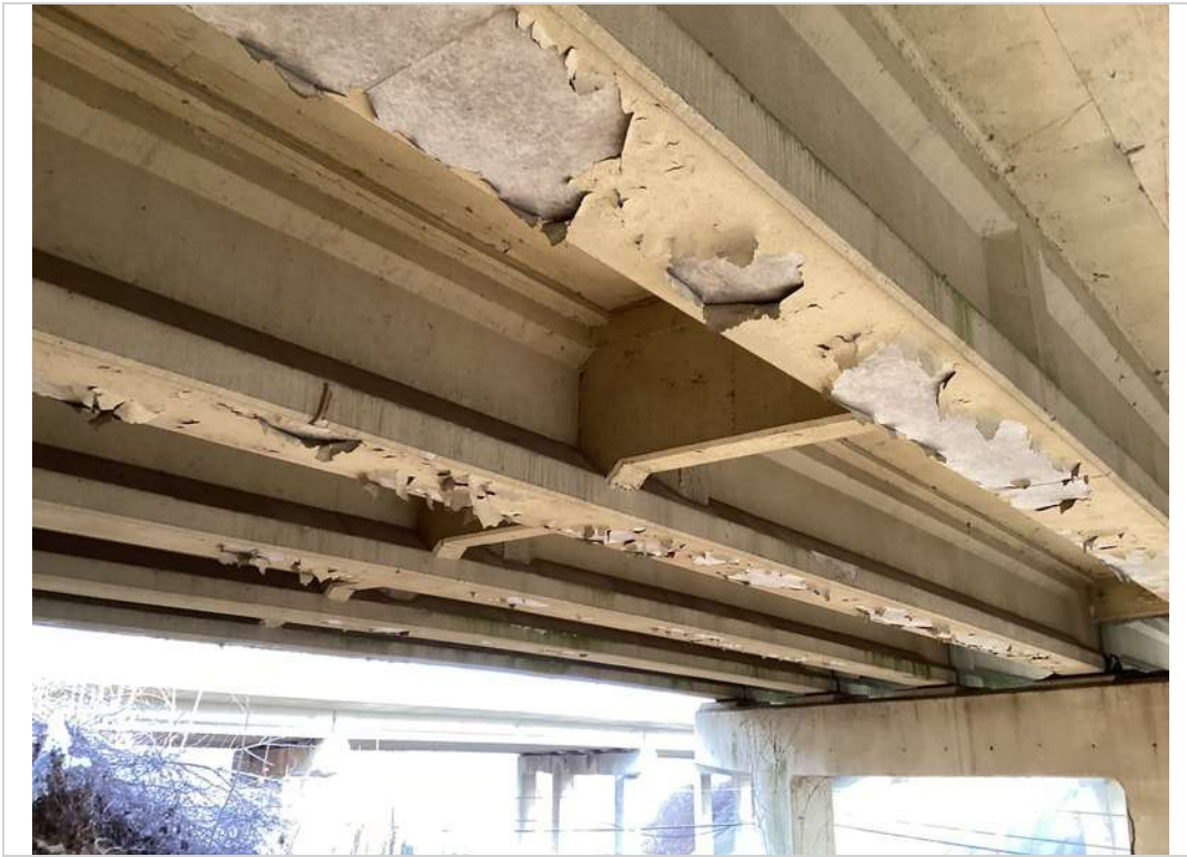
Typical texture coat failure all spans
