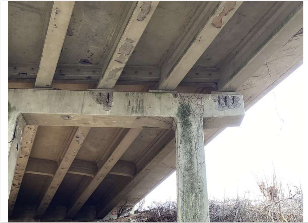
Bent 1 back spalls with exposed rebar
