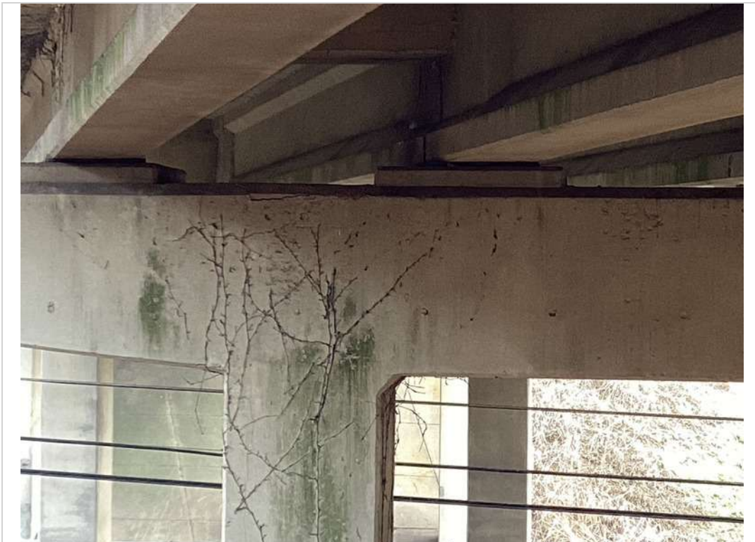
Bent 1 front moderate crack above Column A
