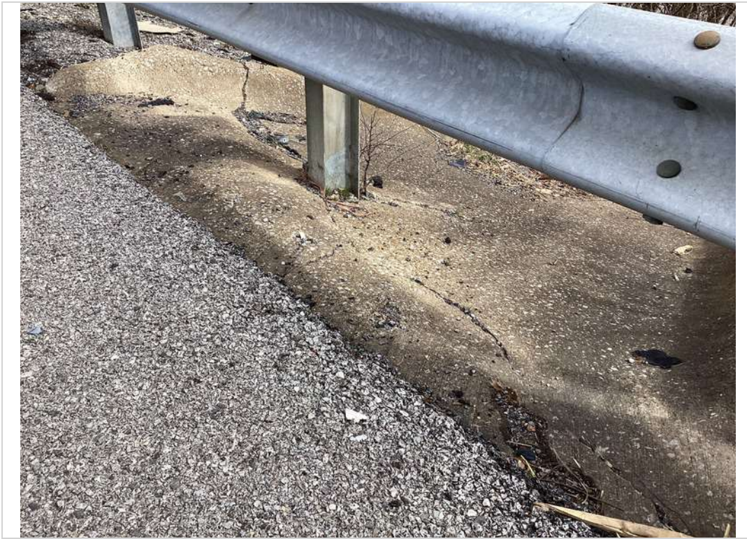
Approach 2 right concrete embankment drain moderate cracks and moderate spall
