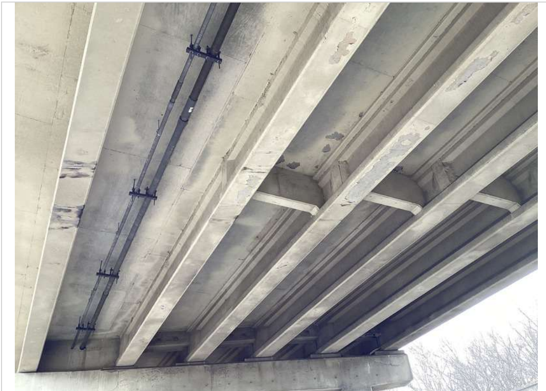
Span 3 collision damage Beams D-F
