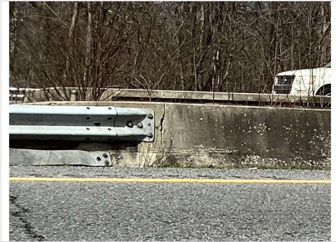
Beginning Span 1 left parapet spall
