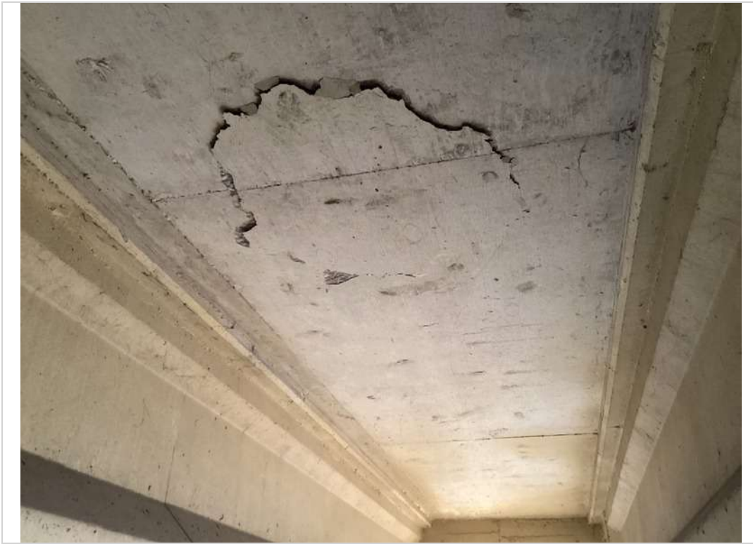
Span 1 Bay B near Abutment 1 delam
