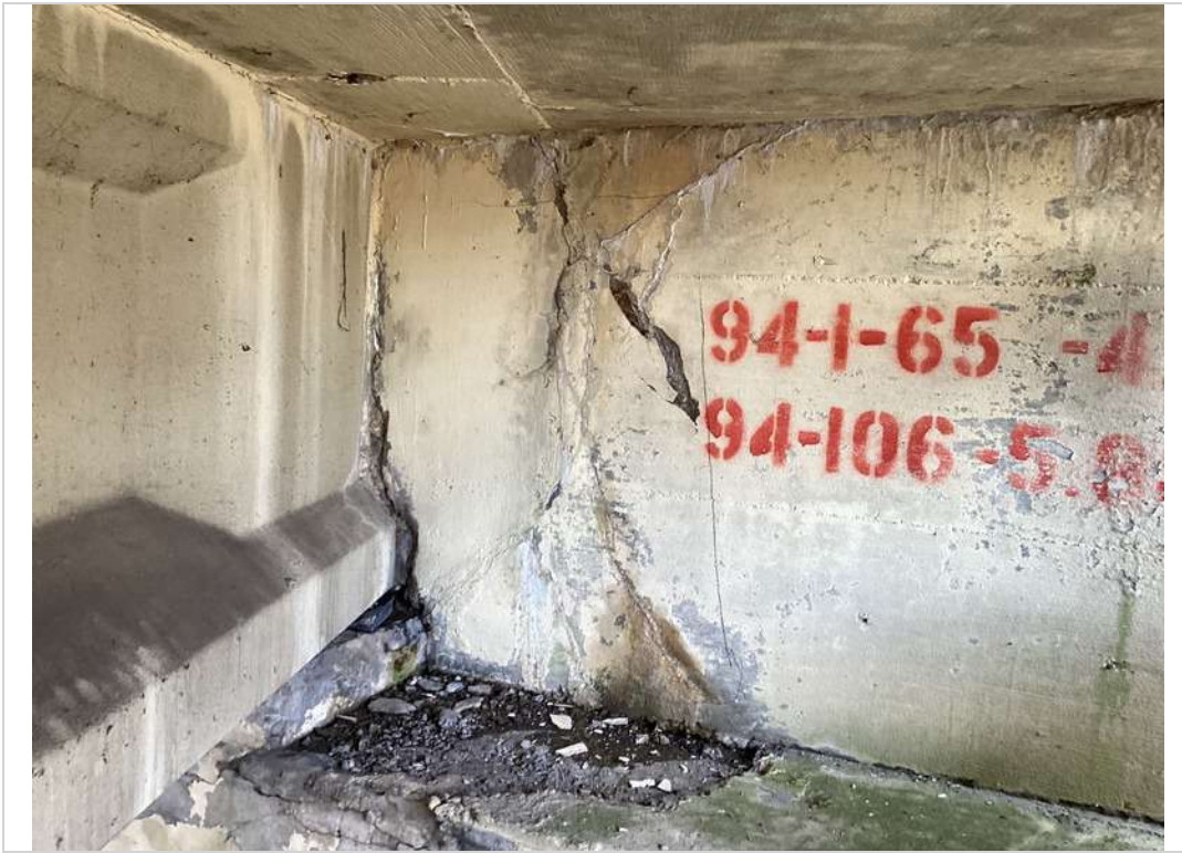
Abutment 1 backwall left of Beam A delam and eff and top of cap spall
