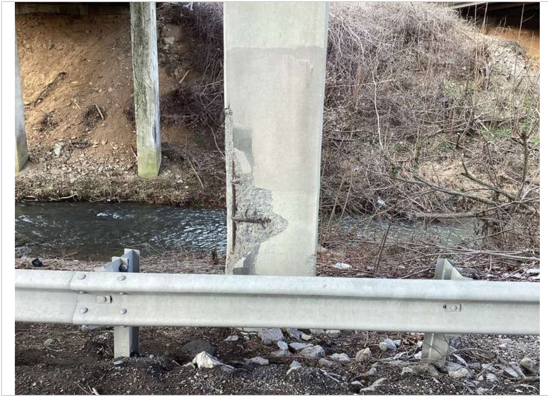
Bent 2 back Column A spall with exposed rebar
