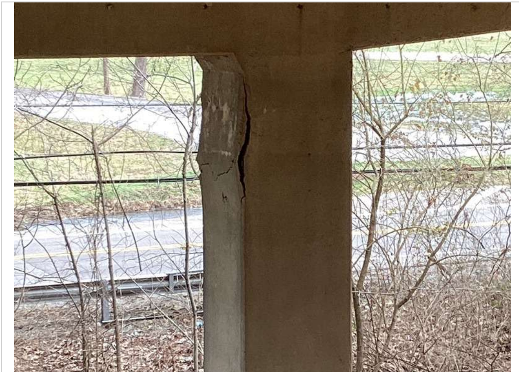
Bent column delam typical
