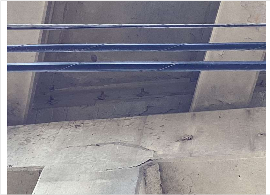
Bent 2 front diaphragms typical moderate cracks on underside
