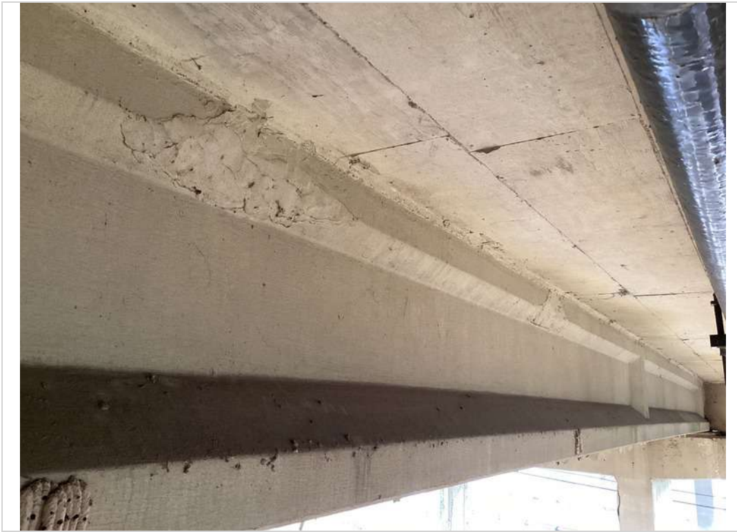
Span 1 Beam E right side top flange patches
