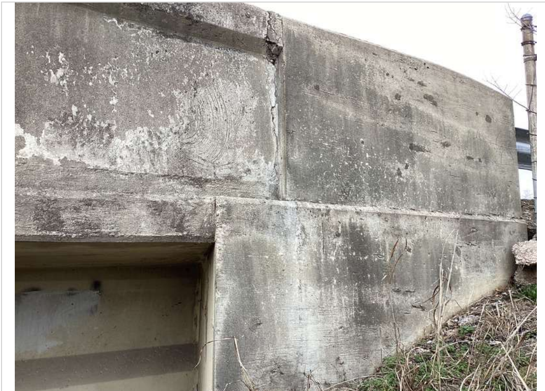
Abutment 2 right parapet over wingwall moderate crack
