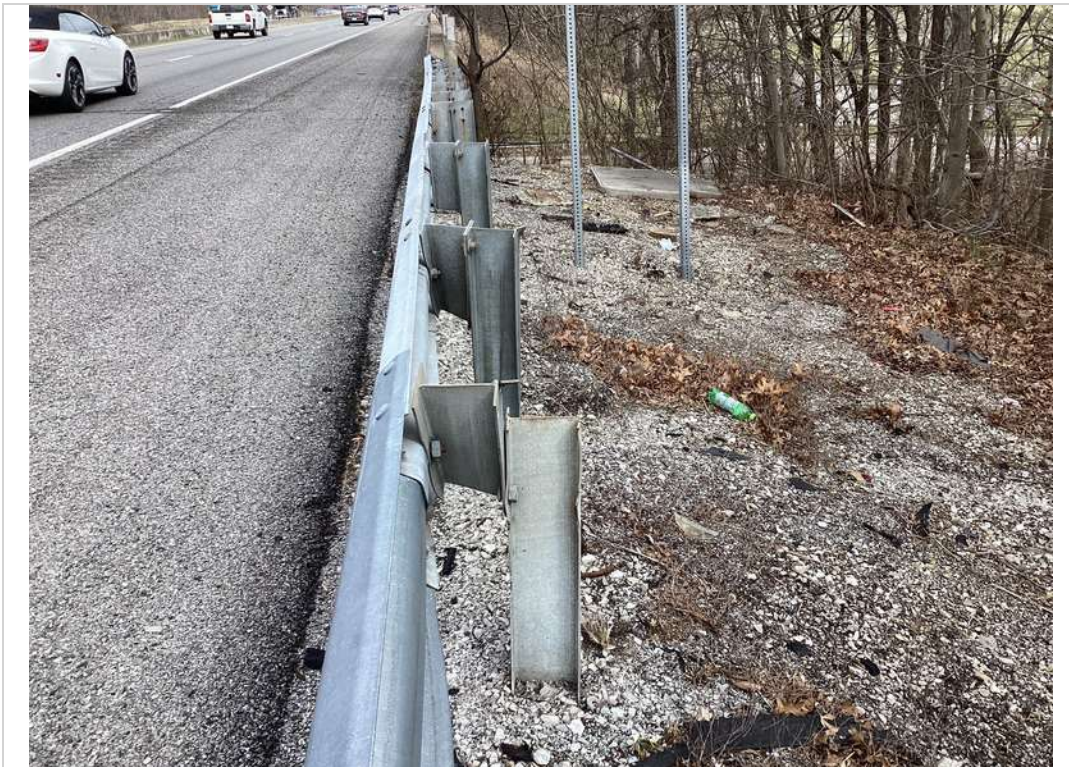
Approach 1 right damaged guardrail posts
