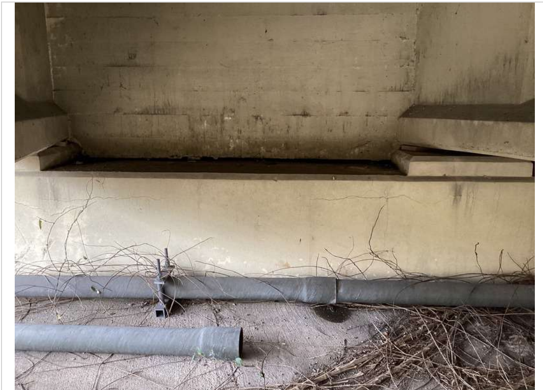
Abutment 2 cap Bay B cracks
