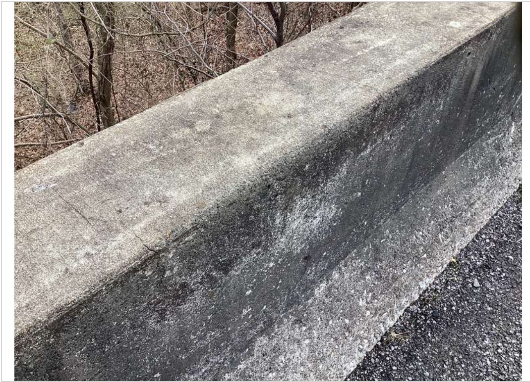
All spans left and right parapet hairline cracks spaced 1'-6" apart
