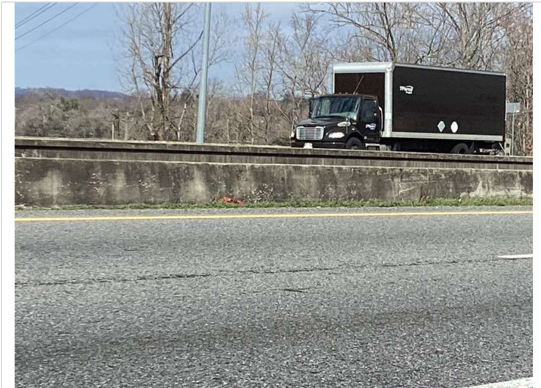
Light vegetation growth along left parapet all spans
