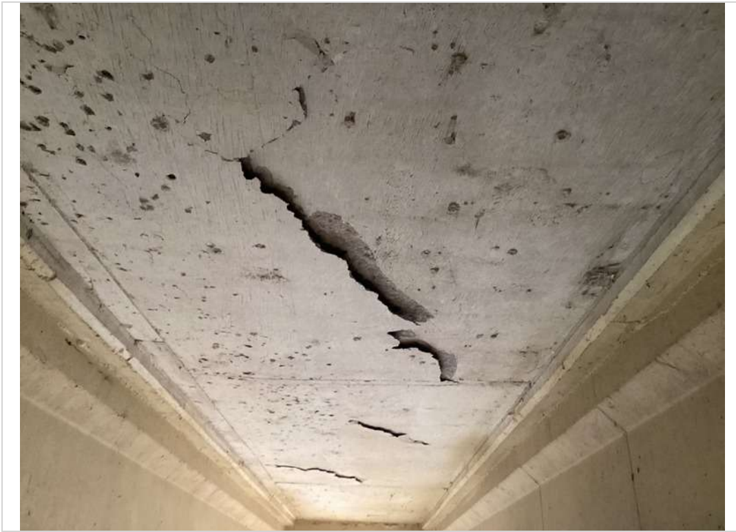
Span 1 Bay A delam from Abutment 1 to midspan
