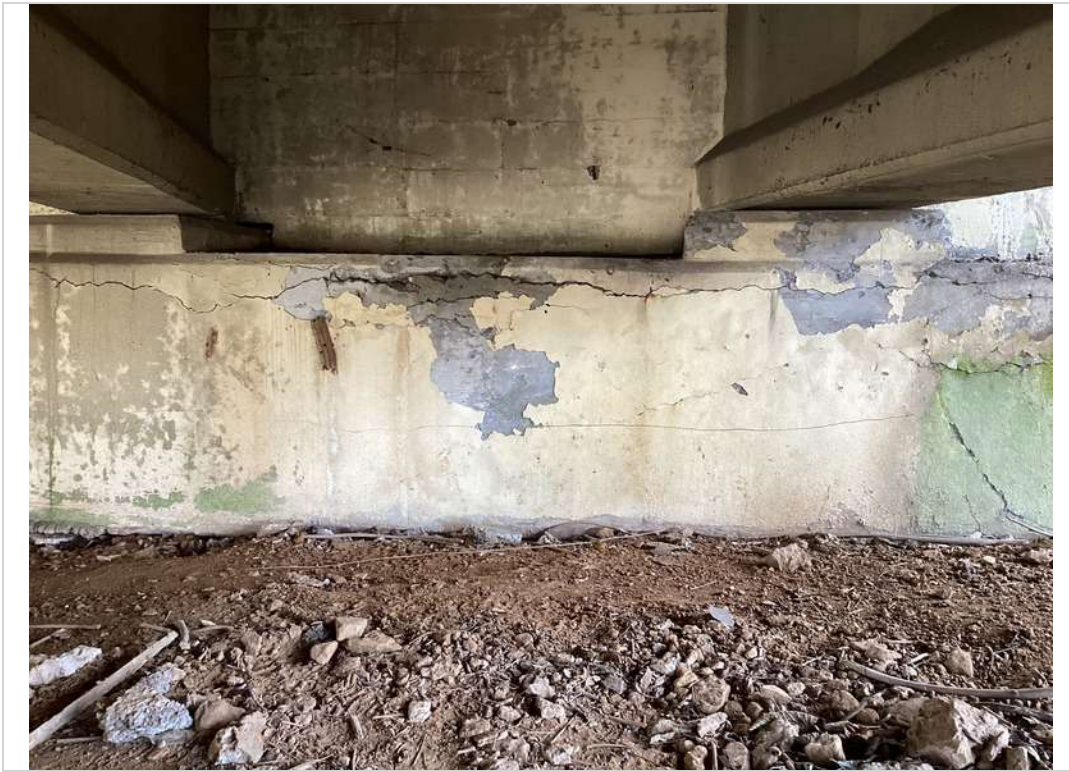
Abutment 1 delam on abutment cap typical throughout
