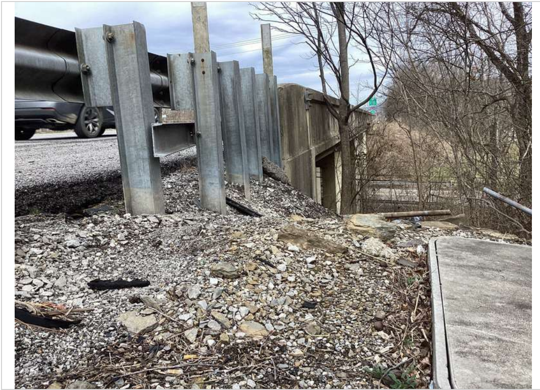
Approach 1 right embankment erosion
