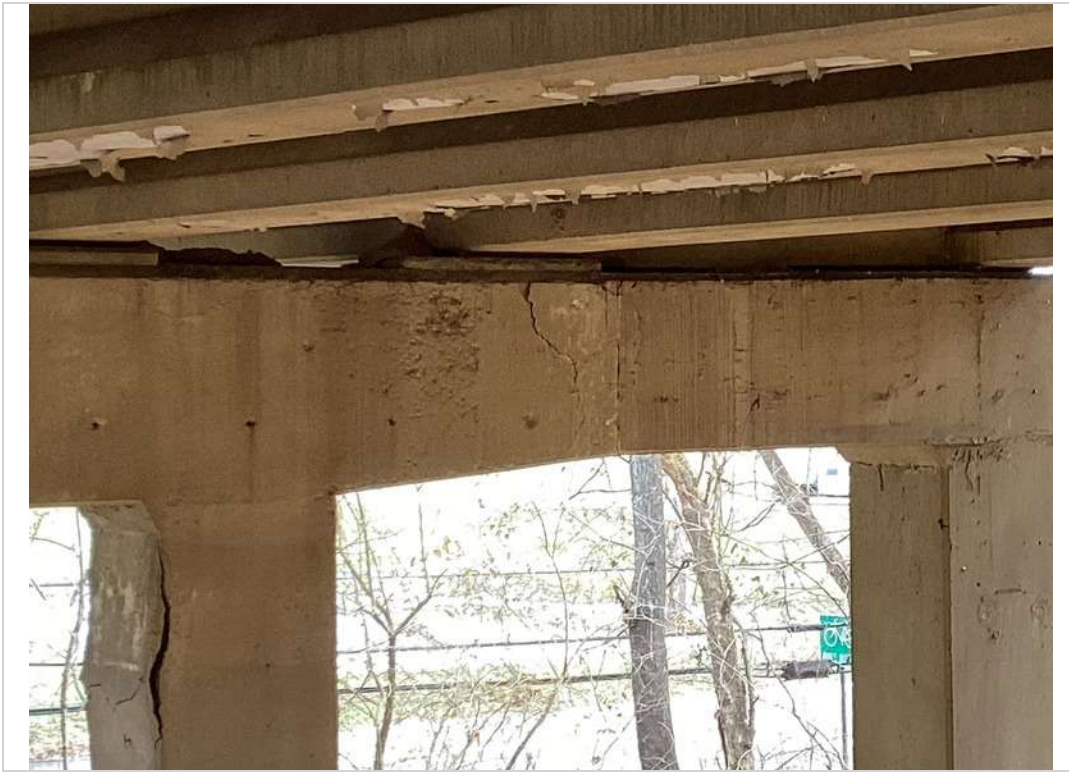
Bent 1 front cap between Column B and C hairline crack, delam, and honeycombing
