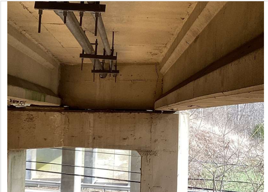
Bent 1 front Bay E diaphragm crack. Typical over Bent 1
