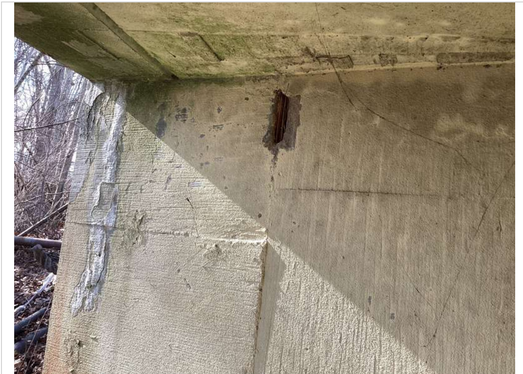
Abutment 1 right end of backwall minor spall with exposed pad between wing and backwall
