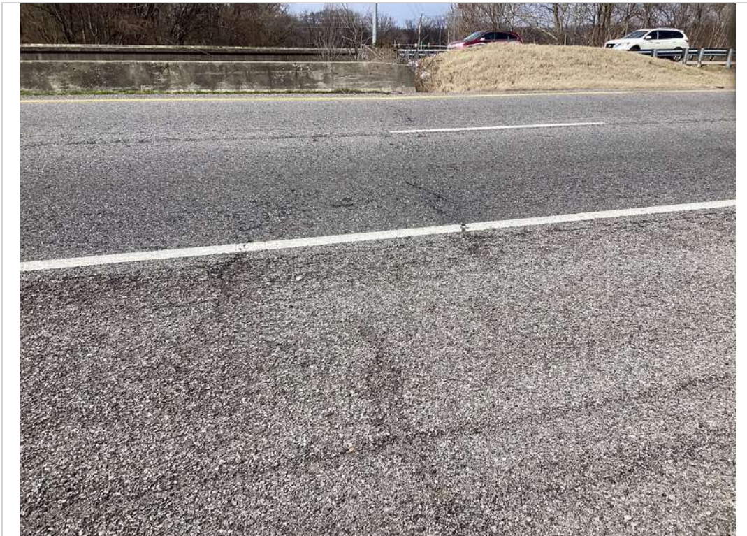
Approach 2 wide asphalt cracks
