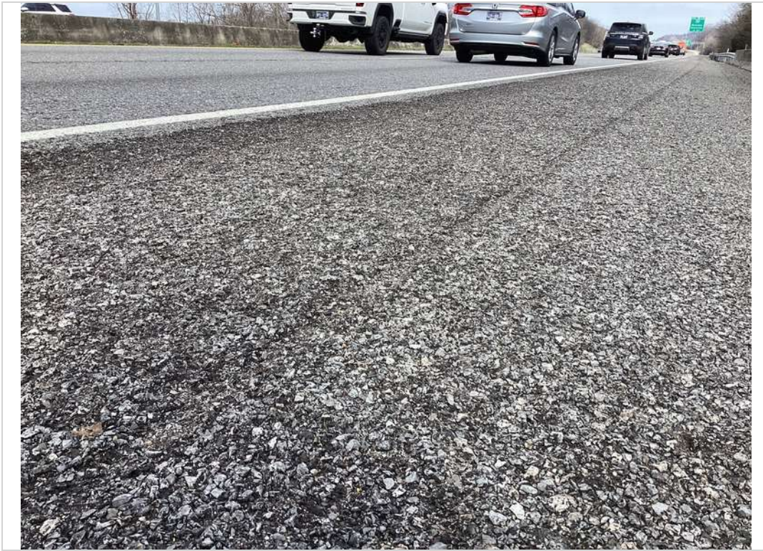
Wearing surface coarse and loose aggregate on right shoulder all spans
