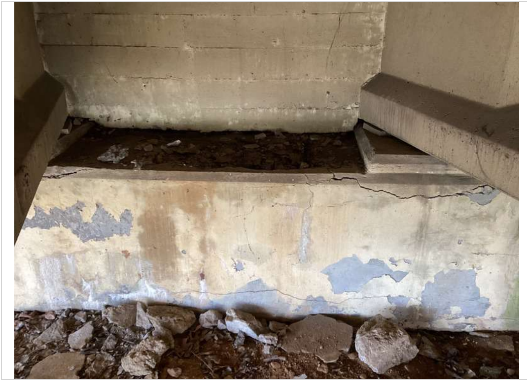
Abutment 1 Bay D crack in cap w/eff and moderate spall with exposed rebar on top of cap
