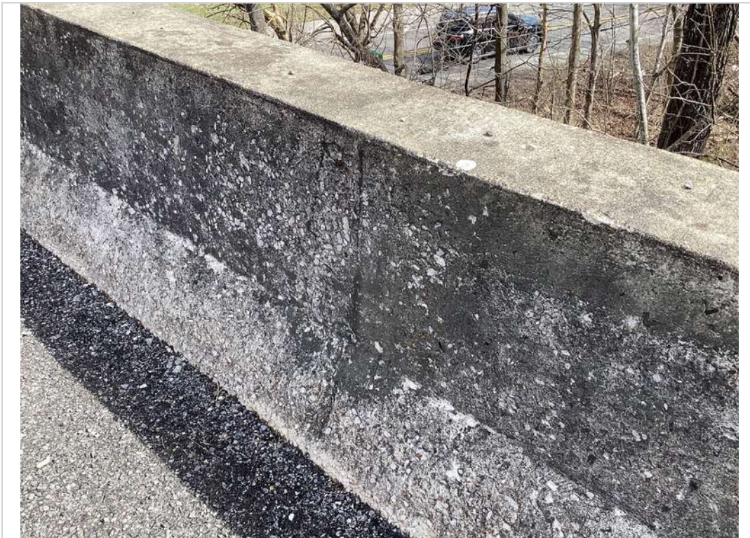
Left and right parapet widespread light scaling with exposed aggregate all spans
