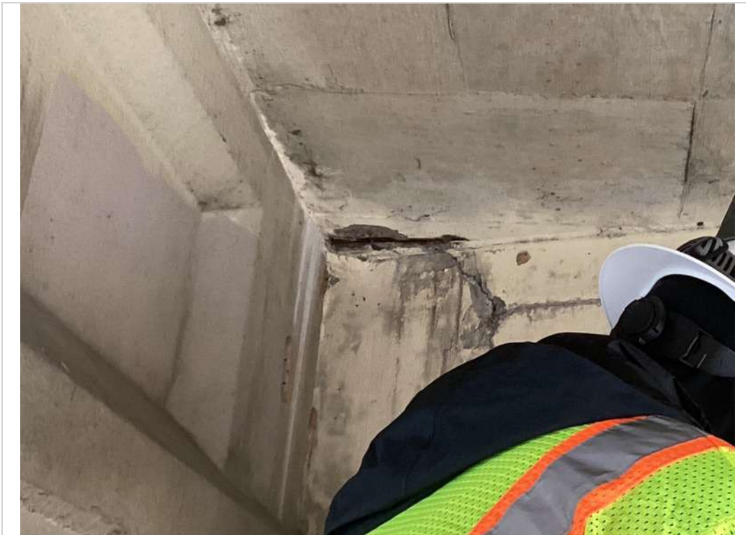
End of Span 4 Bay D spall with exposed rebar
