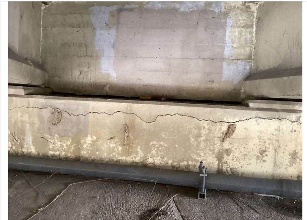
Abutment 2 cap Bay C delam
