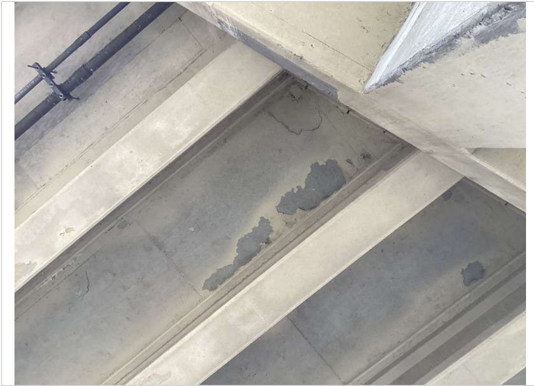
Span 3 Bay D delam
