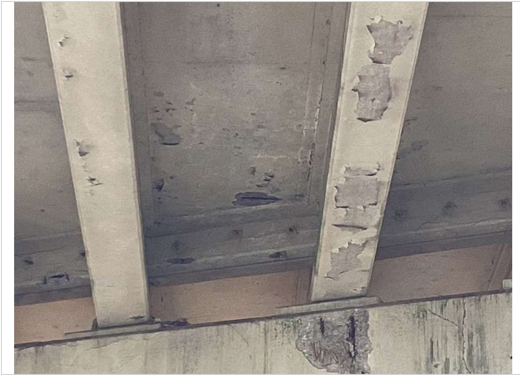
Span 2 Bay C spall with exposed rebar
