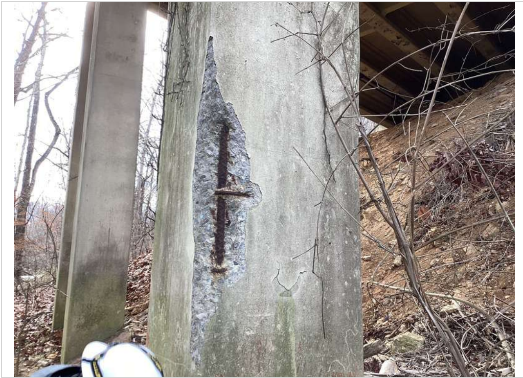
Bent 1 back Column A spall with exposed rebar
