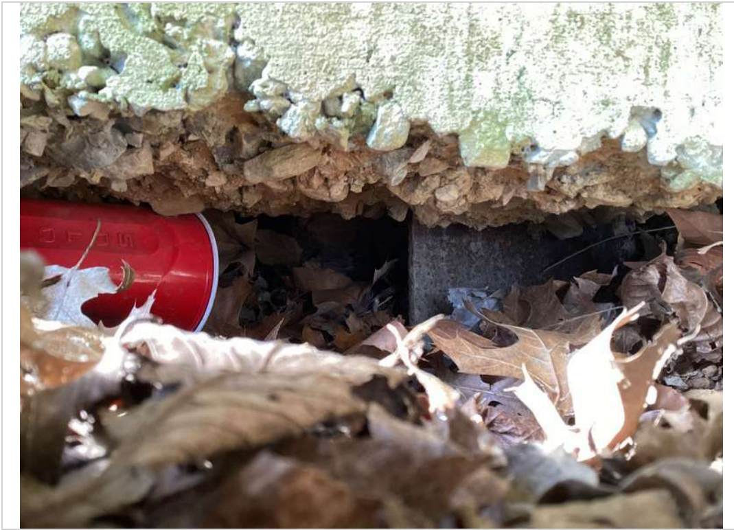
Abutment 1 right end of cap undermining with 1 exposed pile with minor corrosion
