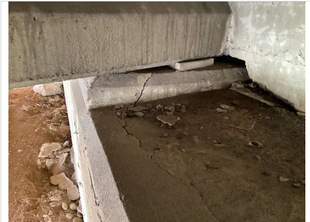
Abutment 1 Riser C crack
