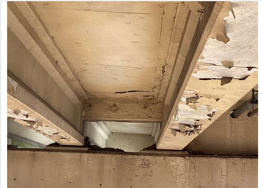
Span 1 above Bent 1 in Bay D delam and diaphragm moderate crack
