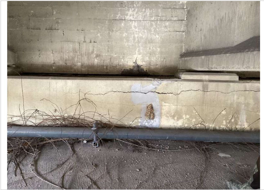
Abutment 2 Bay B cap delam and backwall hairline crack
