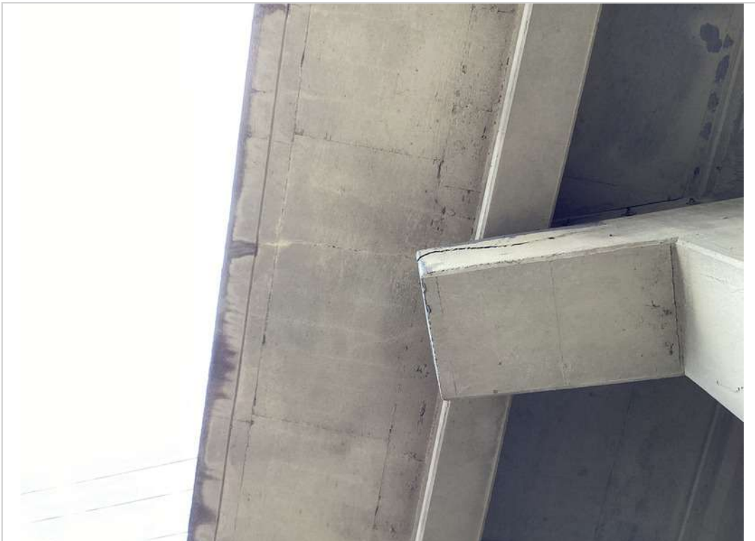
Beginning and end of Span 3 left overhang isolated hairline crack with eff. typical on right overhang
