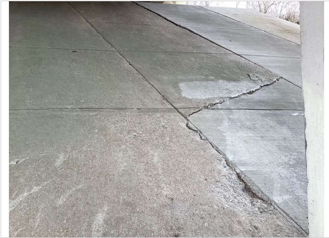
Abutment 2 slope paving typical isolated spall and isolated crack
