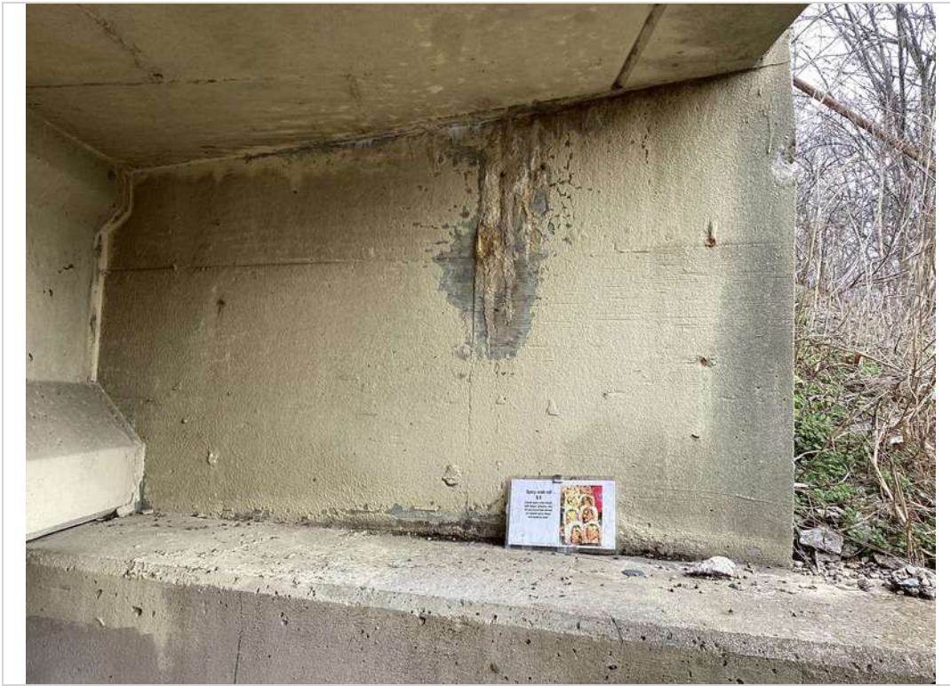
Abutment 2 right end of backwall heavy eff and minor spall
