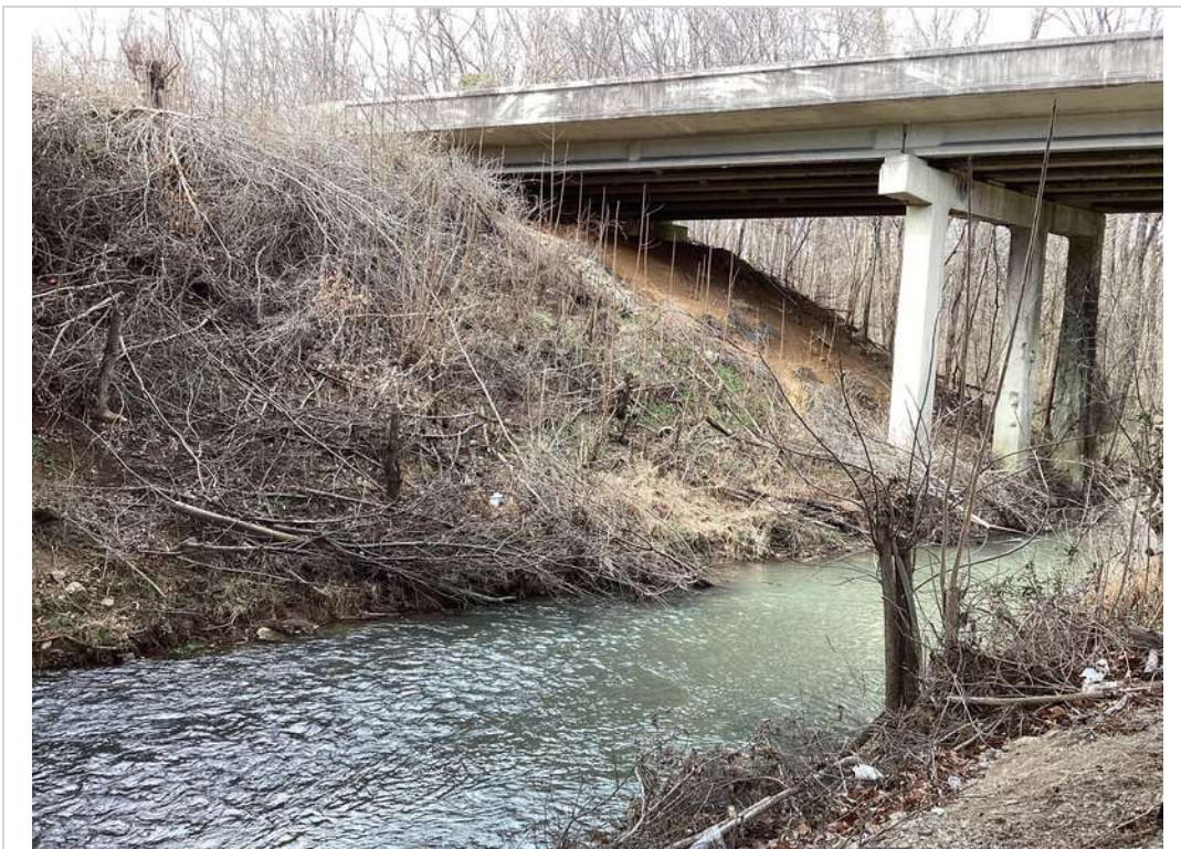
Dead timber debris on Abutment 1 slope
