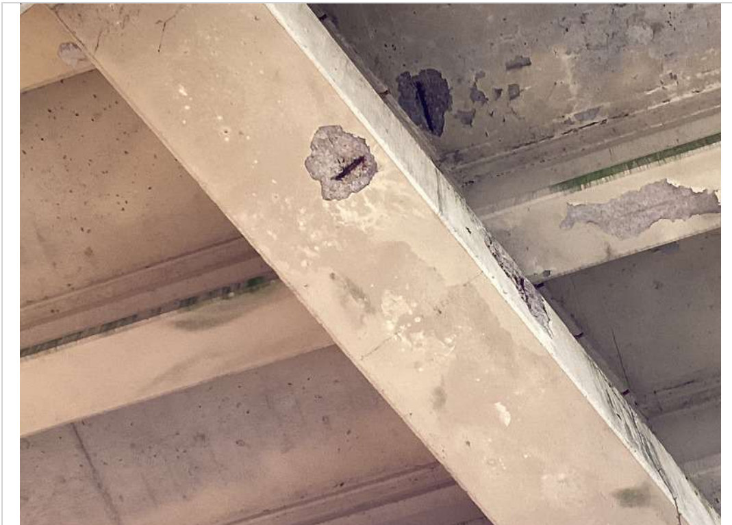
Bottom Bent 1 cap spall with exposed rebar
