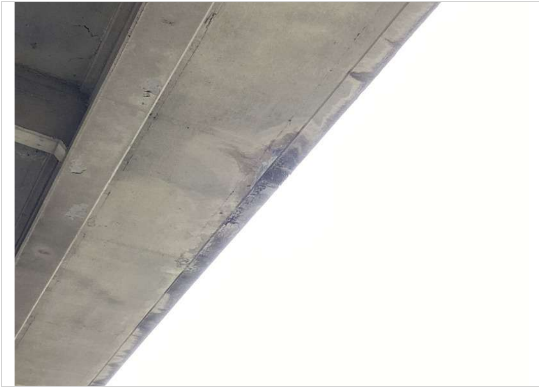
Span 3 left overhang spalls with exposed rebar and water leakage
