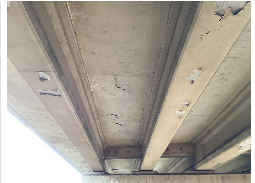
Span 1 Bay A delam from midspan to Bent 1
