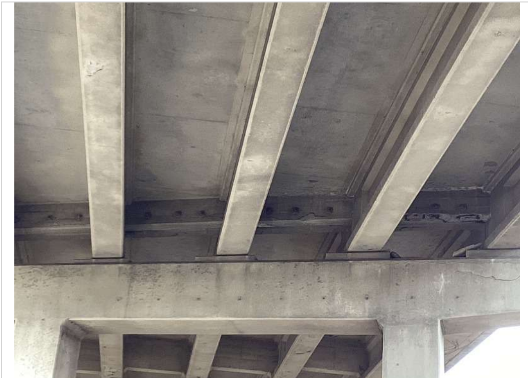
Bent 2 back diaphragms spalls with exposed rebar and delams
