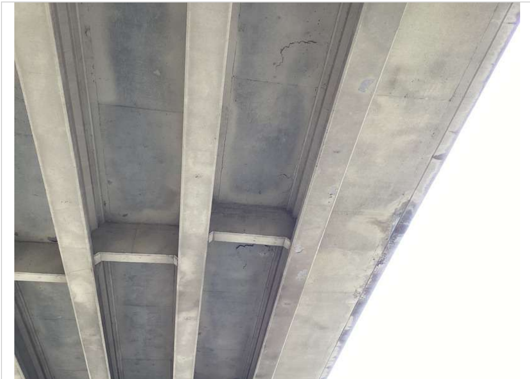
Span 3 Bay A delams
