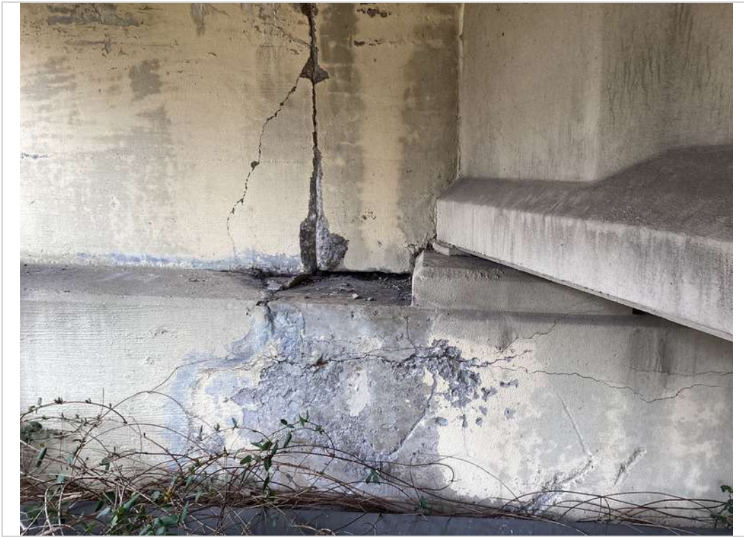
Abutment 2 backwall and cap left end cracks, spalls, and delam
