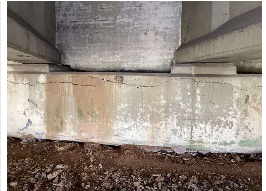
Abutment 1 Bay B delam Bay B and undermining
