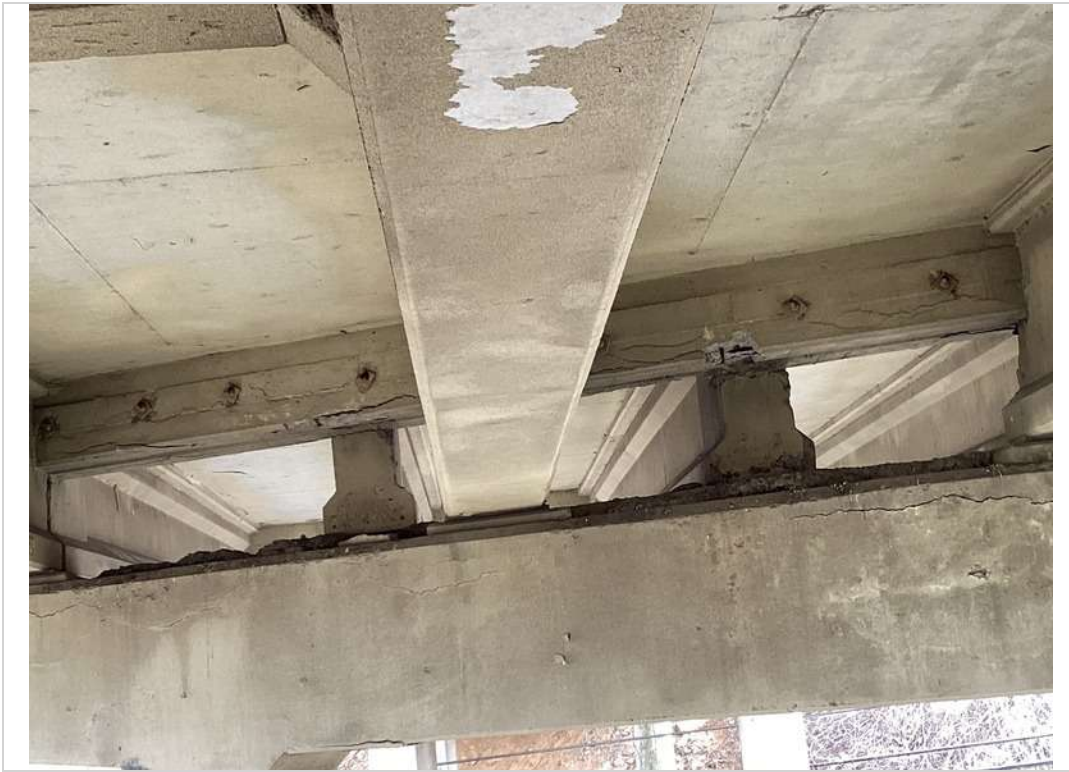
Bent 3 back typical diaphragms delam and spall with exposed rebar
