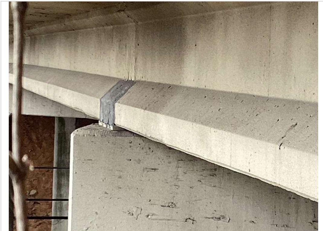
Beginning Span 4 Beam E cracked patch in bottom flange
