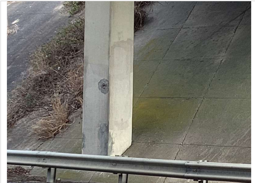
Bent 3 front Column A spall with exposed rebar
