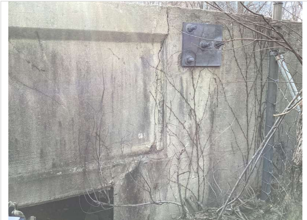
Abutment 1 parapet and wingwall crack typical both sides
