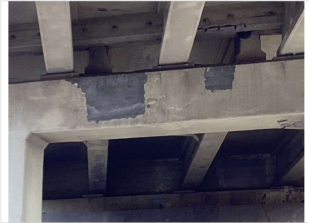
Bent 3 front typical unsound patch with eff
