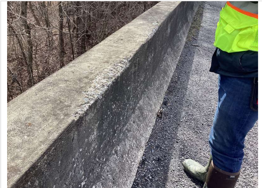
Span 1 right parapet spalls
