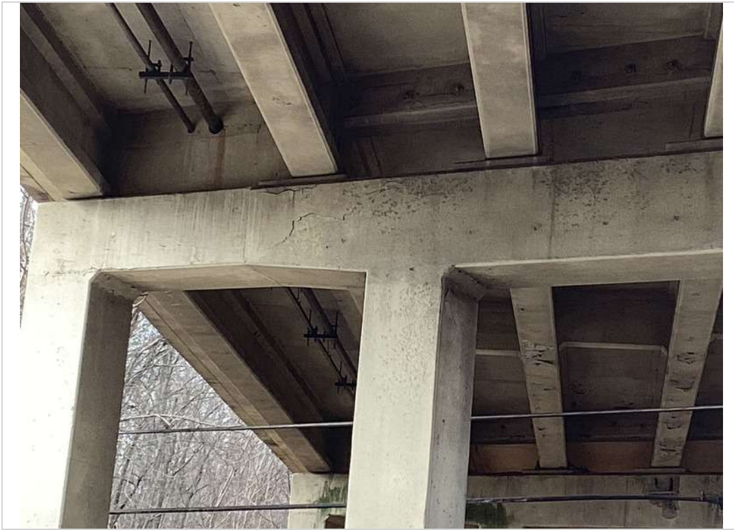
Delam in bent cap typical
