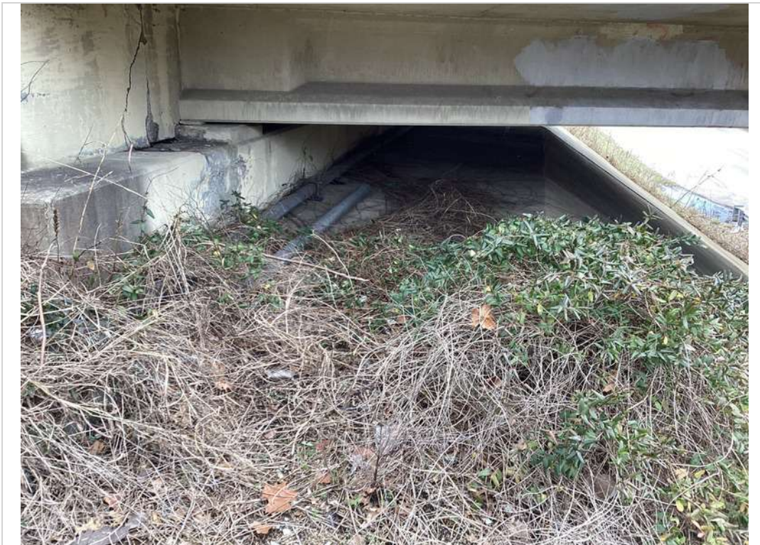
Abutment 2 left end slope paving vegetation growth
