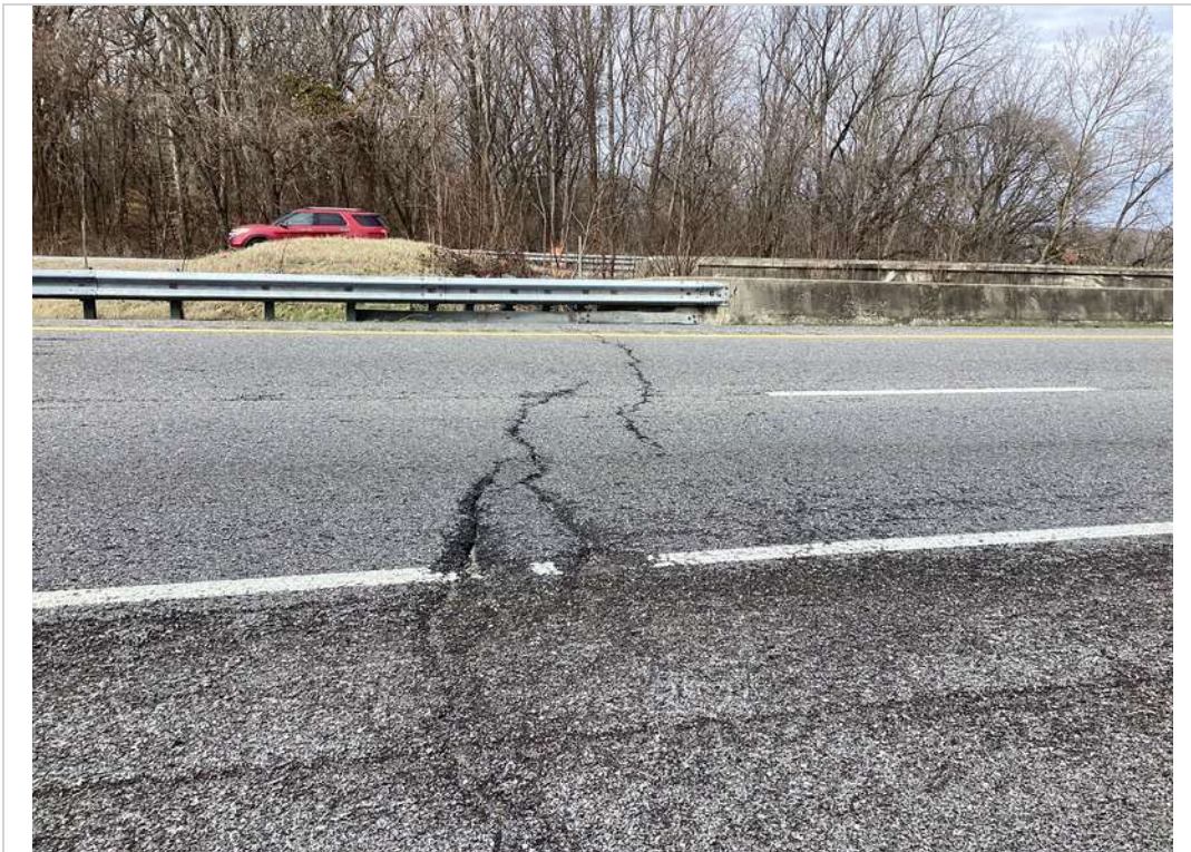
Approach 1 wide asphalt cracks and moderate potholes
