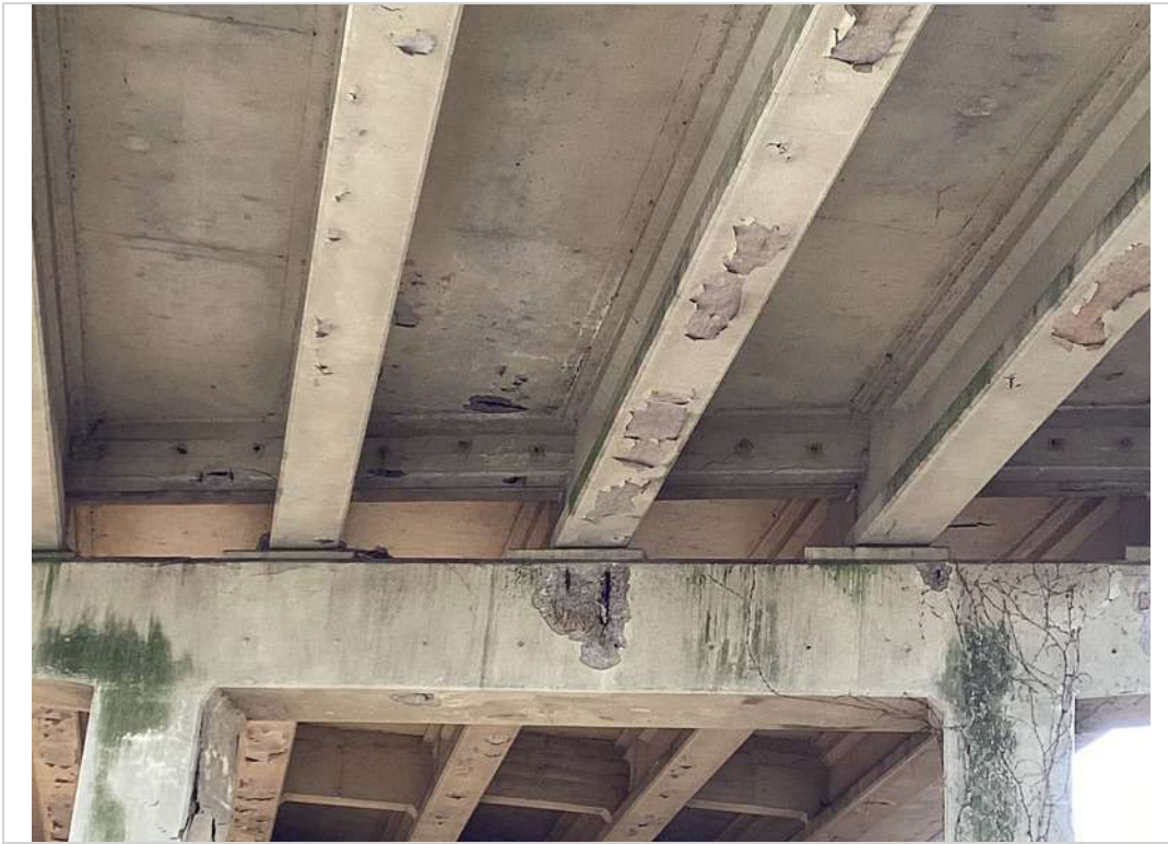
Diaphragms over back of Bent 1 some spalls with exposed rebar and moderate cracks
