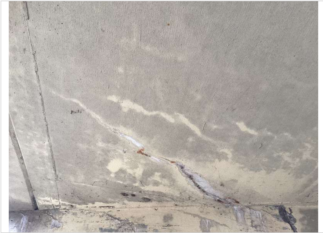
End of Span 4 left overhang hairline cracks with eff
